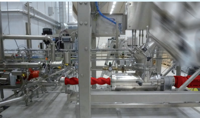
The MX 30R progressing cavity pump was customised for use in the dough mixing process at Isernhäger. Image: Isernhäger
